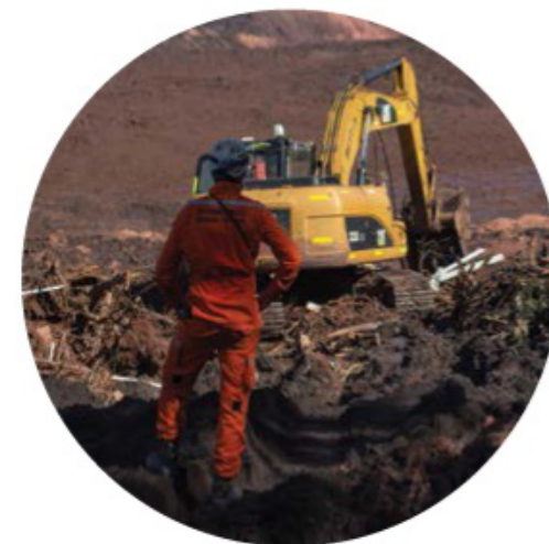
Minas Gerais firefighters conduct a search operation at Corrego do Feijao in Brazil, after a dam collapsed at an iron ore mine belonging to mining company Vale near the town of Brumadinho in Brazil in January 2019.
